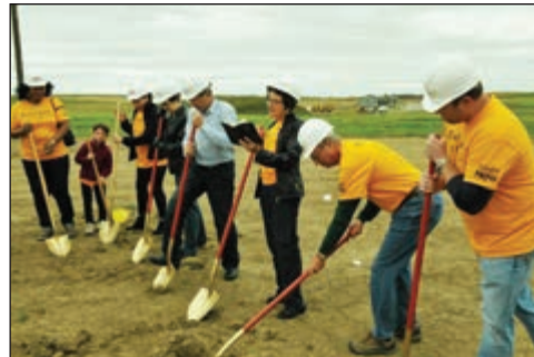
Members of WestSide Lutheran, Sioux Falls, break ground for their church building in September 2013.
